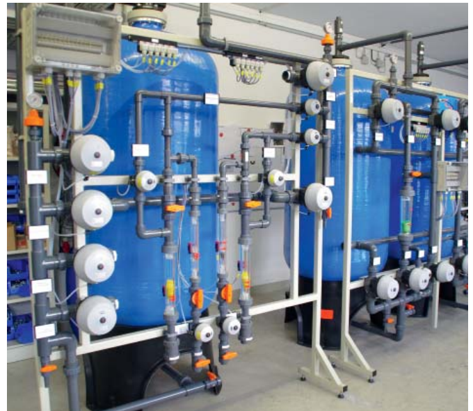
Ion exchangers and gravel filtration plants
